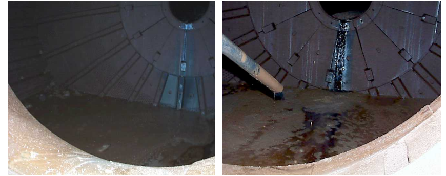
Figure 9: Crash Stop Charges at 425 (left) and 450tph (right)
